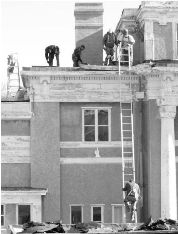
October 2008: Work on installing a new roof begins on the Sanborn House.
